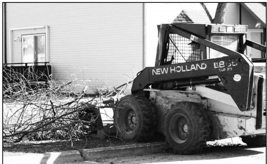
Belling Tree Service employees work swiftly and safely while removing branches from yards.
